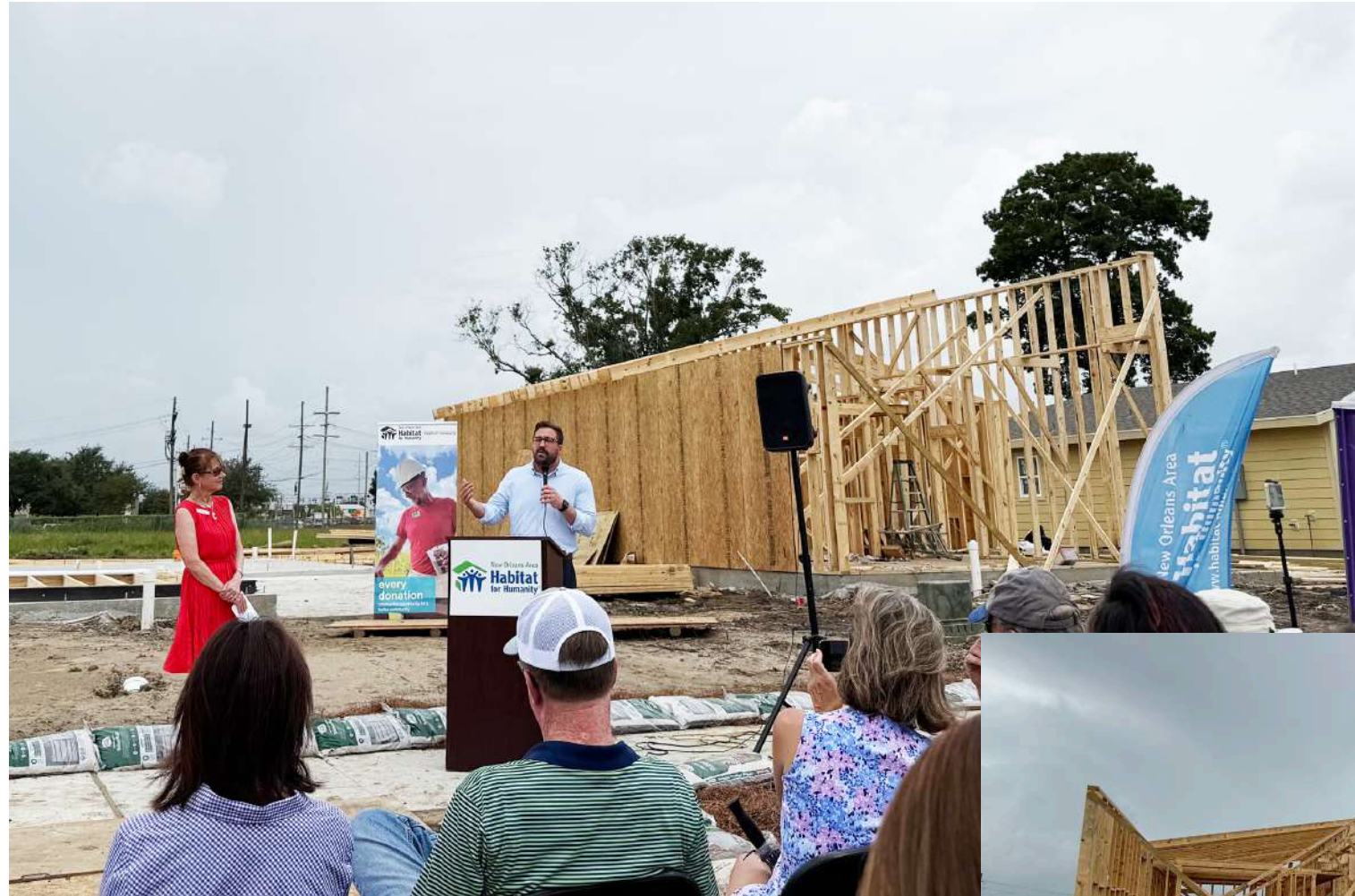
Construction underway for homes in the Rising Oaks community in Terrytown, Louisiana.
